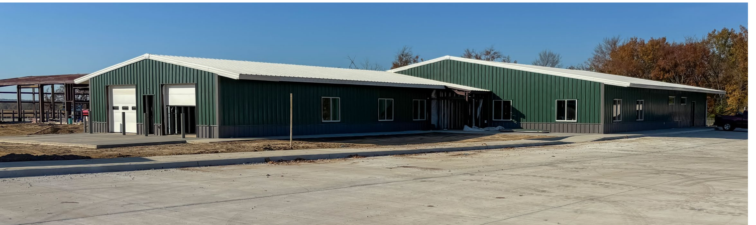
Construction is underway for the new facility in District 1 and is set to be completed in Summer 2026.
