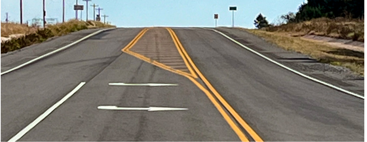
Facing East: A hill on SH-39 creates limited visibility for drivers approaching the SH-102 junction from the east, which is why the new left turn lane and shoulders at this location are essential for driver safety.
