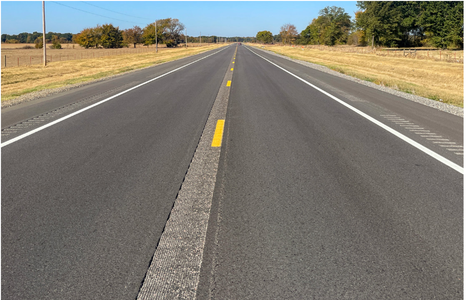
After: The final section of this SH-3 corridor is complete with new pavement, shoulders and rumble strips.
