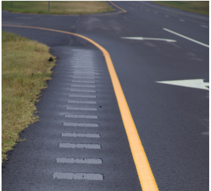
A rumble strip's vibration and noise is designed to alert drivers that their vehicle is leaving the travel lane.
