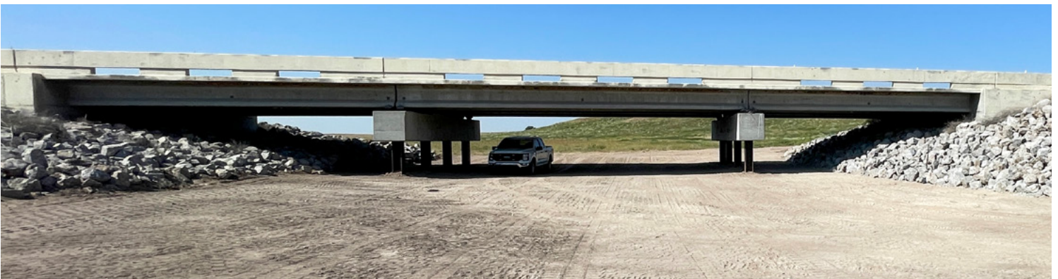
Filling the scour hole took three-hundred cubic yards of material to achieve. District 6’s crews completed this job in less than one month.
