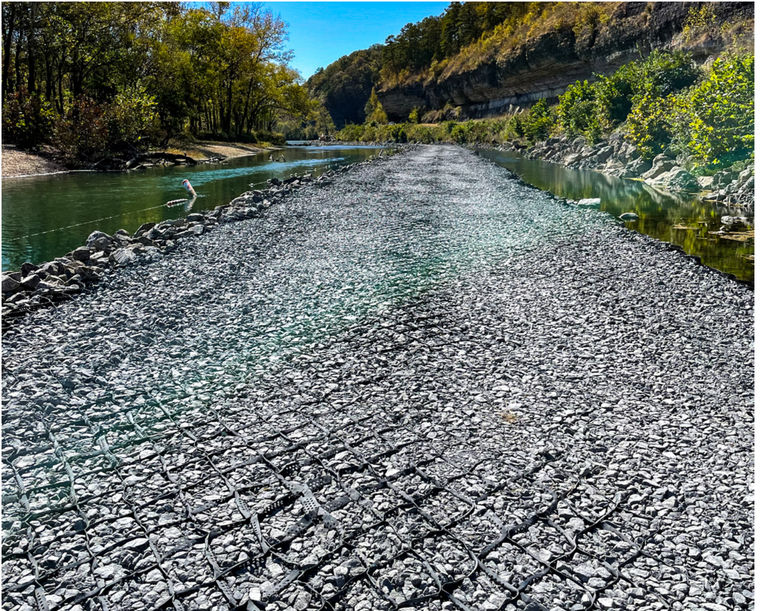
The retaining wall in the Illinois River was constructed to combat erosive effects on its slopes.
