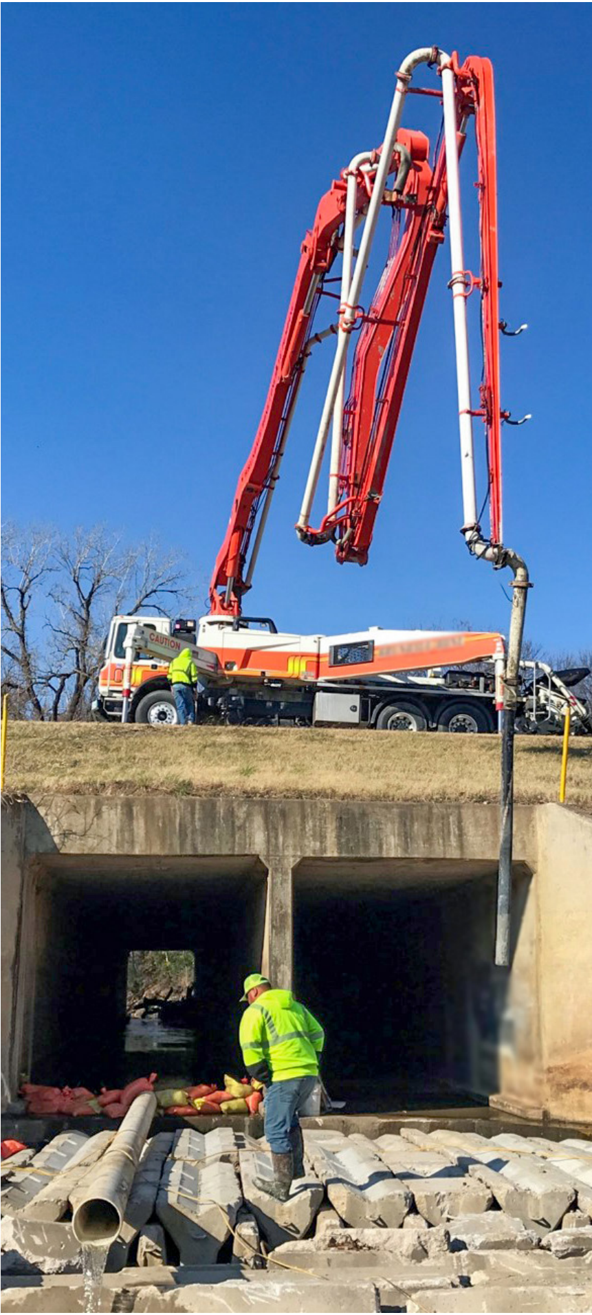
A maintenance crews in District 8 works to repair a downstream scour hole under a reinforced concrete box bridge.
