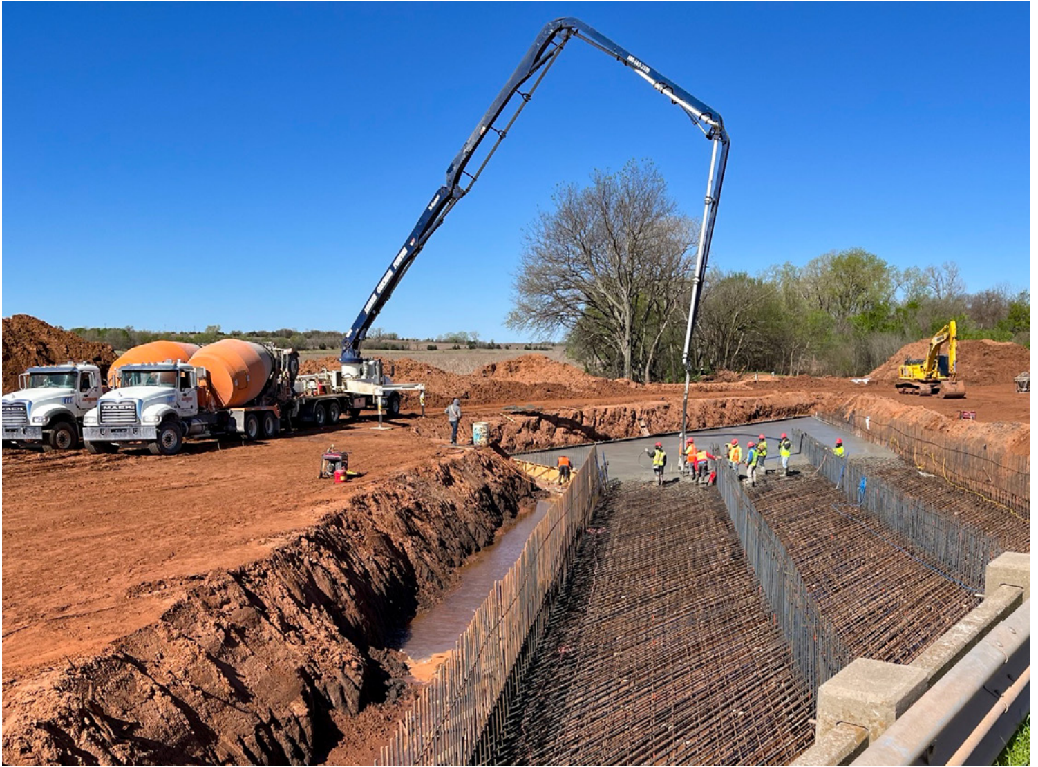
A crew lays concrete for a culvert with a concrete pump truck.
