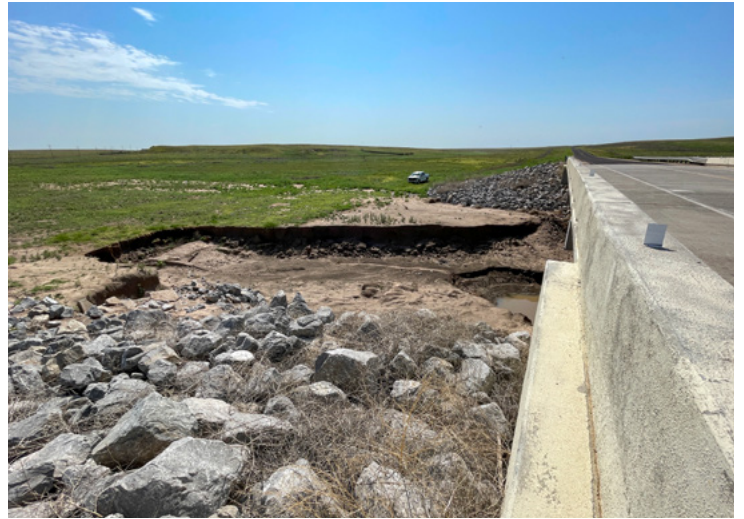
Bridge scour happens when underwater sediment is washed out from under a bridge’s foundation.
