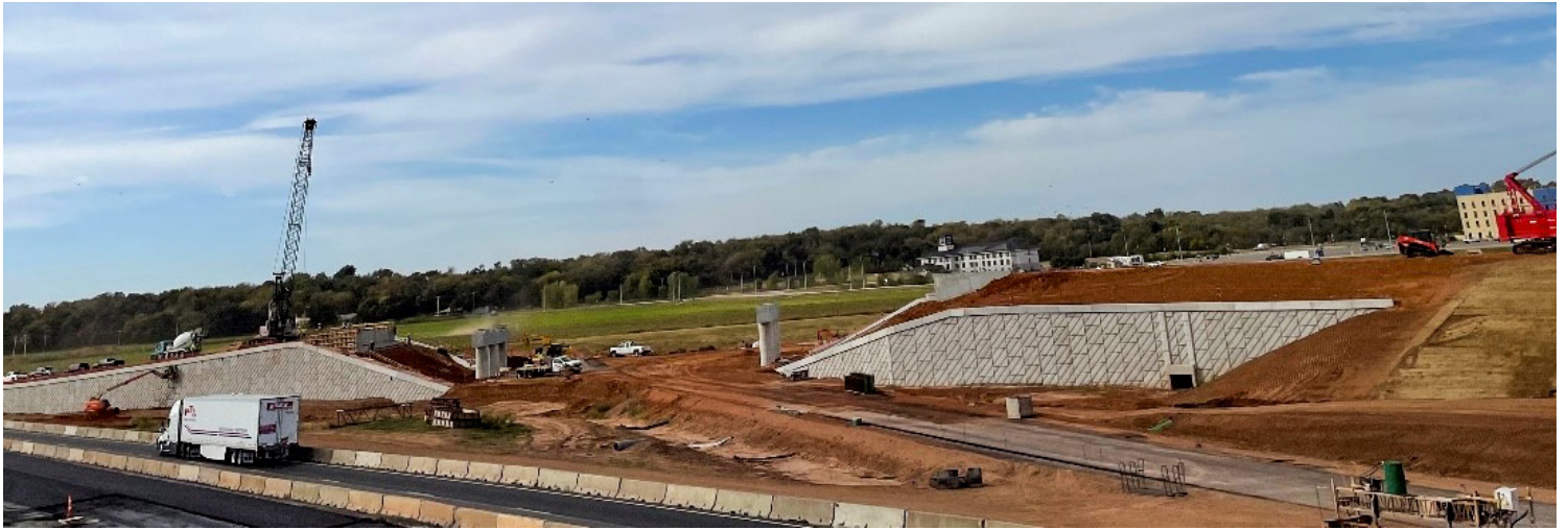
A wide angle of ongoing construction for the new SH-9/I-35 junction in Cleveland County.
