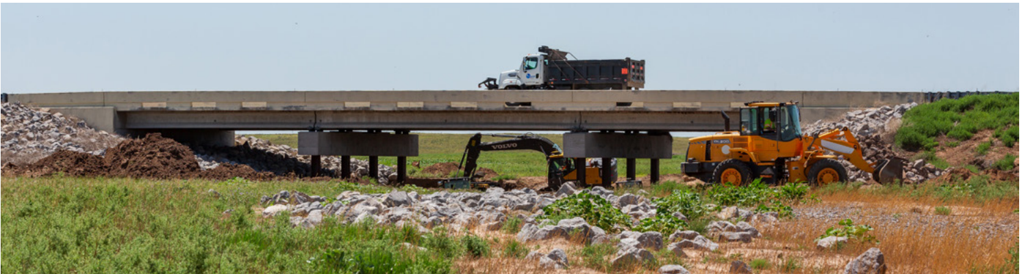
District 6’s maintenance crews work to fill and compact the scour hole with materials.
