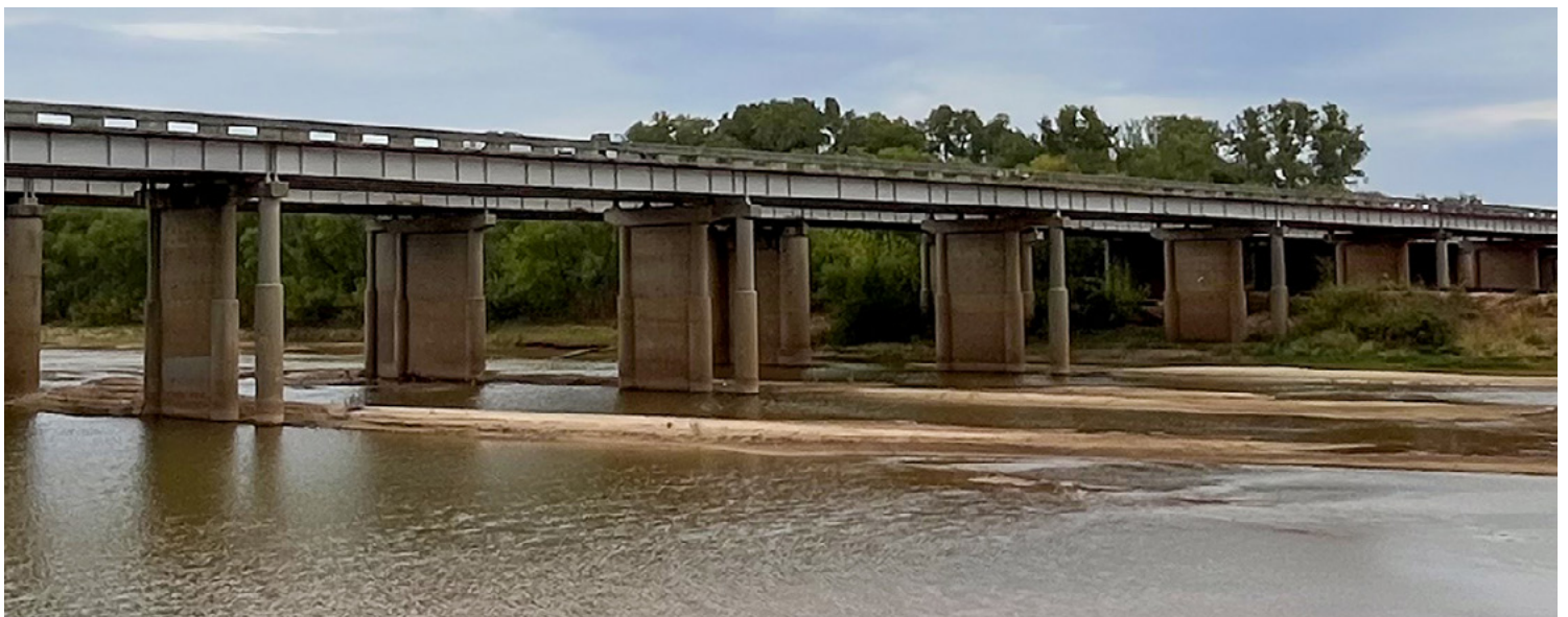
A close-up view of the I-35 bridge substructure taken from the Texas side of the Red River.
