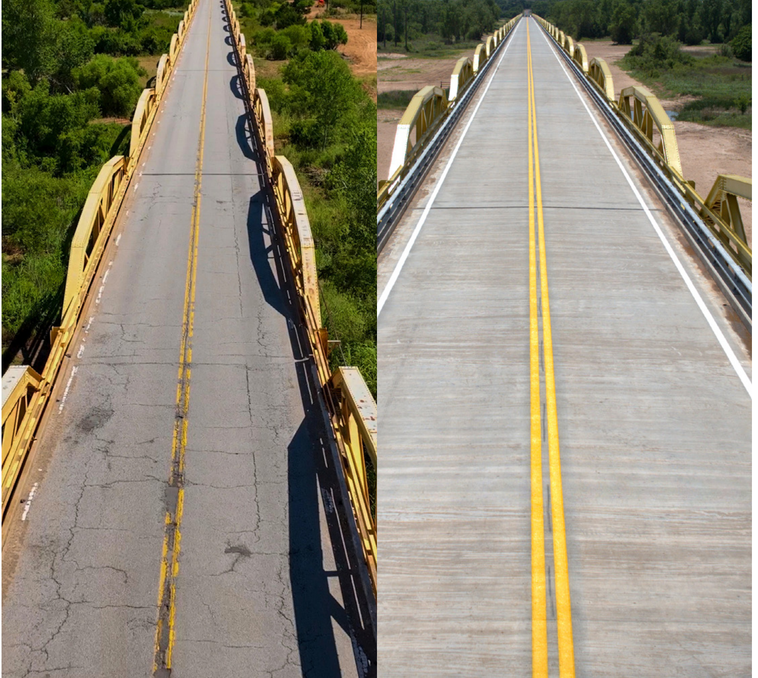
Bridgeport – A comparison of the Route 66 Bridgeport bridge's condition before (left) and after (right) its restoration.
