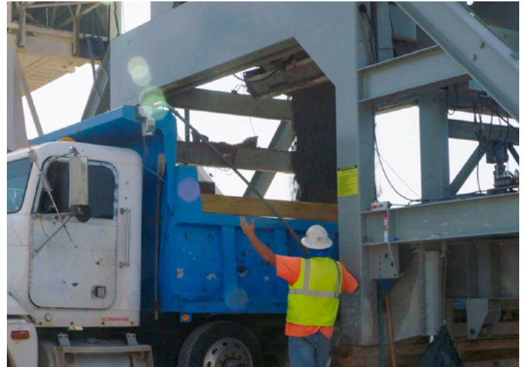
Materials drop into the back of a dump truck, while a crew member signals to the truck driver.
