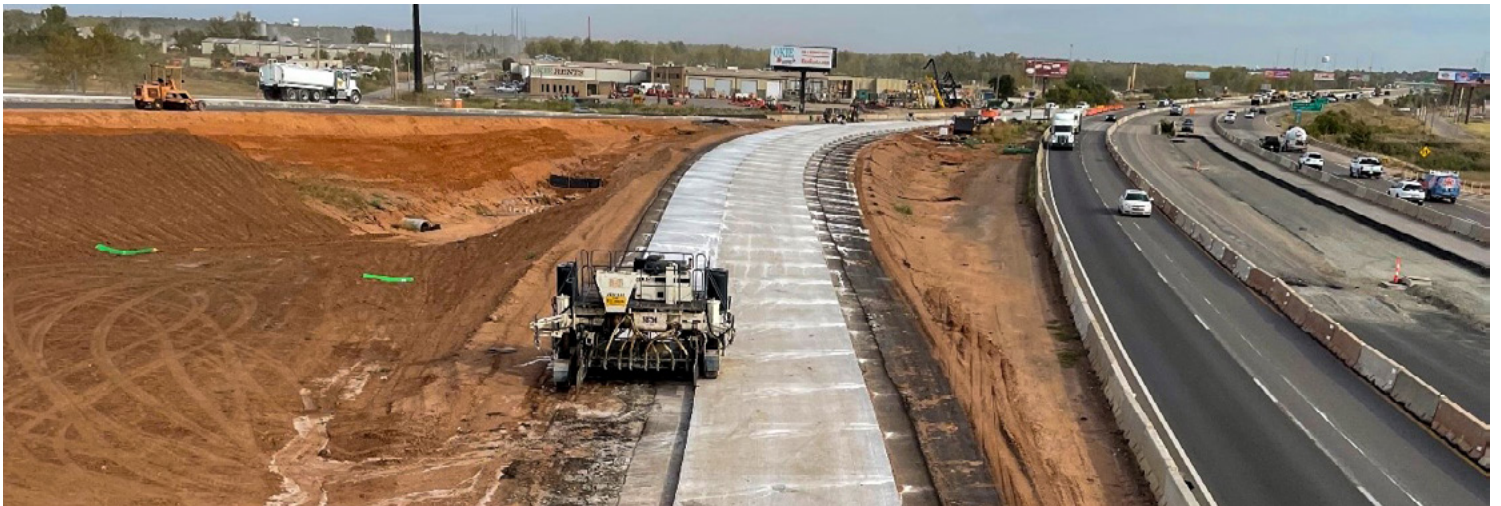
Paving and other heavy operating equipment in motion next to I-35 southbound traffic.
