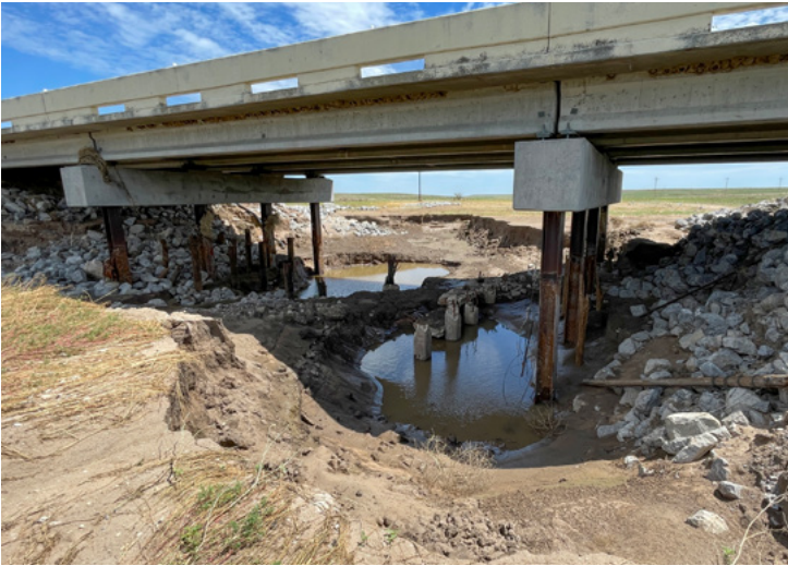
Under the Three Seeds Draw Creek bridge, water fills the 12-foot-deep scour hole.
