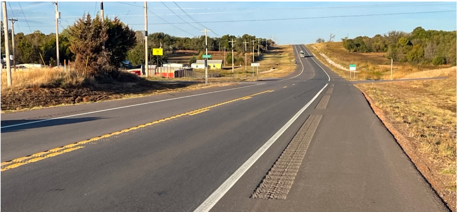
Facing West: New shoulders on SH-39 at the Grady and McClain County line.
