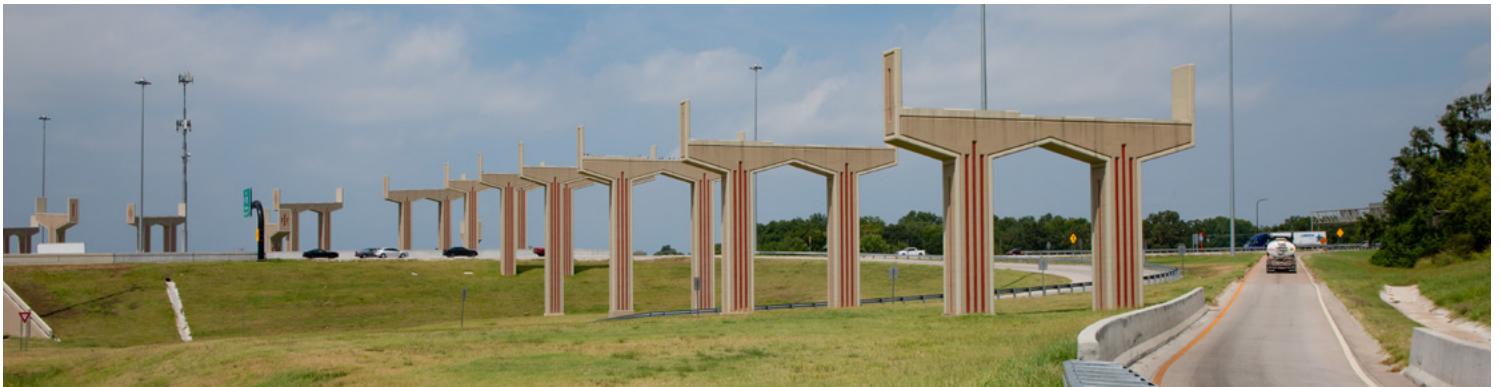
Phase 2 of the I-44/US-75 interchange in Tulsa will soon be underway. Pictured are bridge abutments that are locally referred to as, ODOT's Stonehenge.
