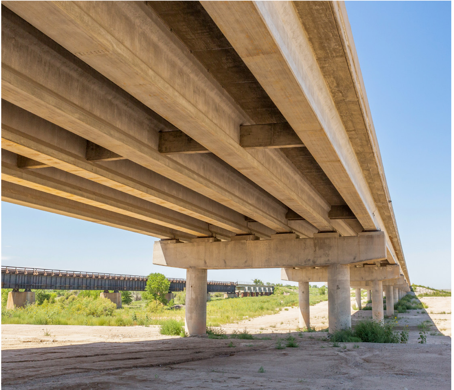
A view of US-287's new substructure over the Cimarron River north of Boise City.
