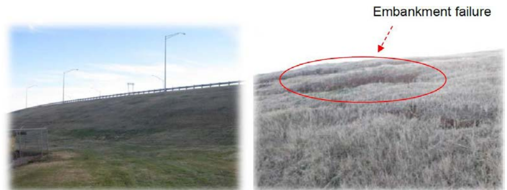
Figure 1 Failed slope of a highway embankment in Chickasha, Oklahoma
