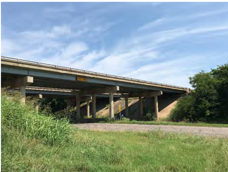
Photograph 4: NBI# 15735 (US-69 NB) over Ark St and K.R.R., recently painted and no swallows observed.
