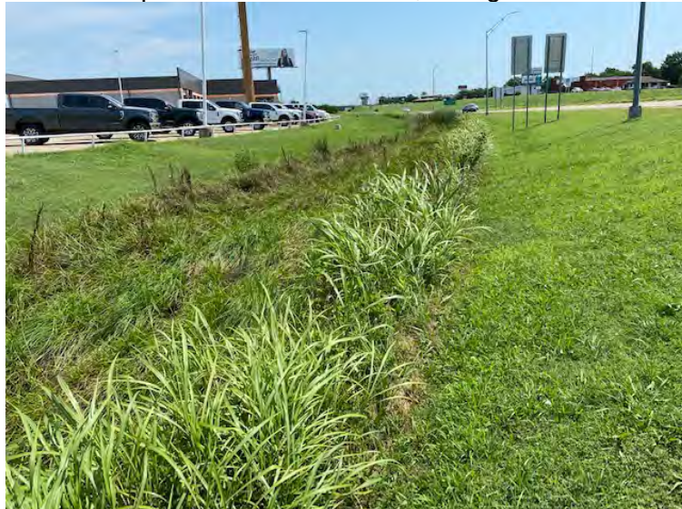
Photograph 20: R4SBC-02, continued on west side of US-69 SB off ramp, facing north.
