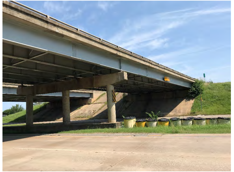
Photograph 7: NBI# 17507 (US-69 NB) over Main St, recently painted and no swallows observed.
