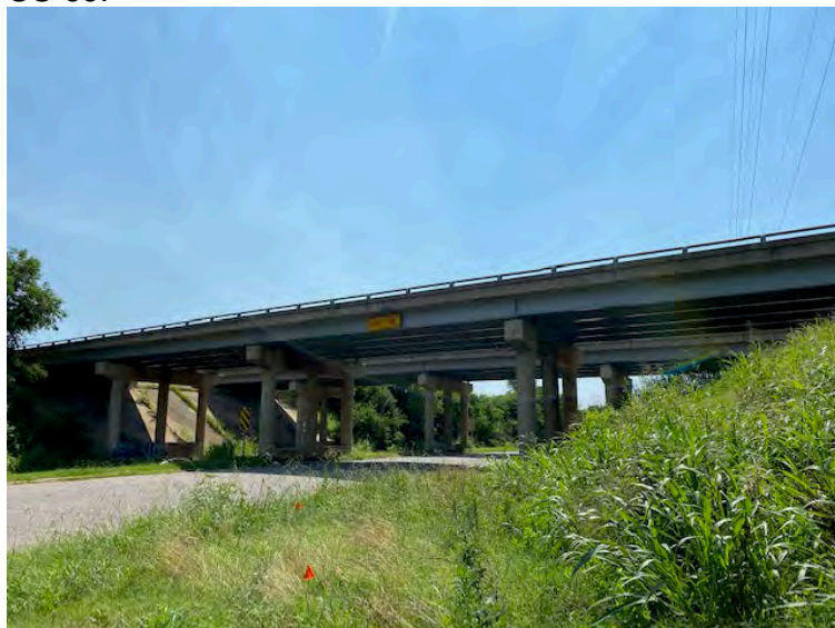
Photograph 5: NBI# 15734 (US-69 SB) over Ark St and K.R.R., recently painted and no swallows observed.
