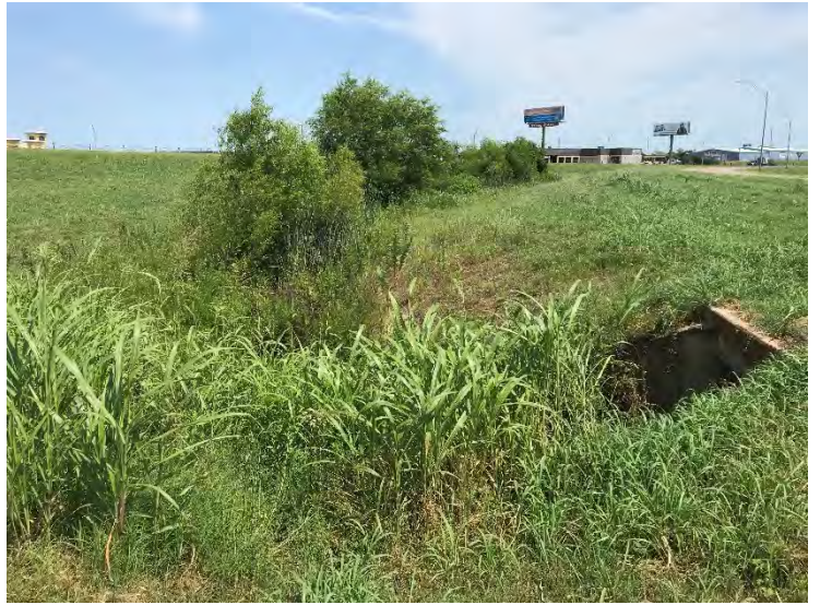
Photograph 17: R4SBC-02 observed in between on and off ramp to northbound US-69, facing north.
