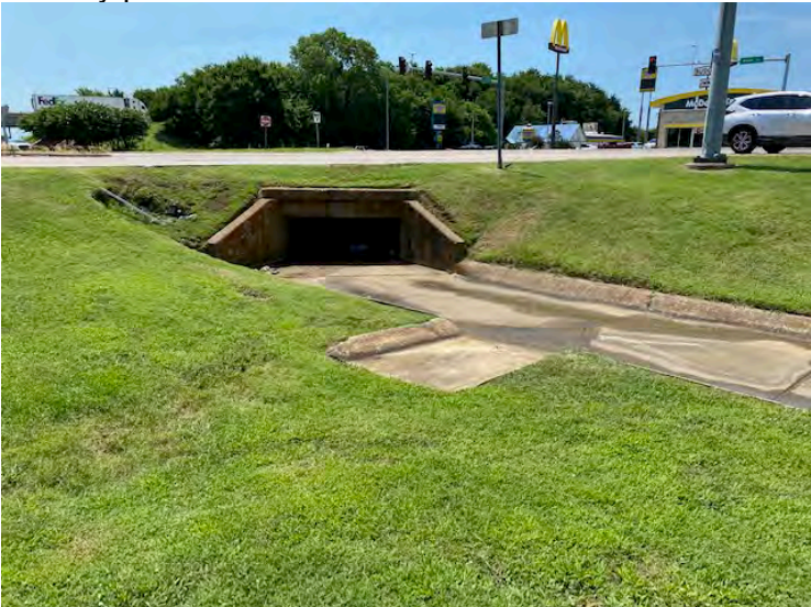
Photograph 10: Structure #6 and start of NDF at west corner of west US-69 SB off/on ramp and Main Street. No swallows observed.
