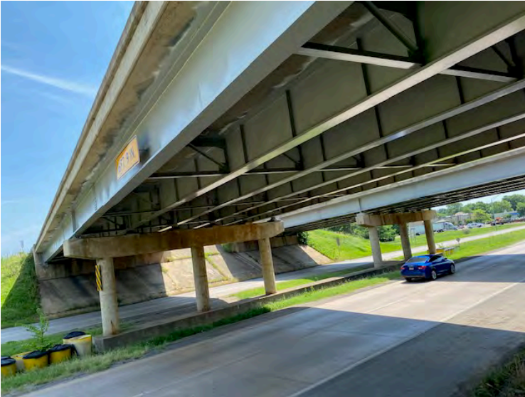
Photograph 8: NBI# 17506 (US-69 SB) over Main St, recently painted and no swallows observed.
