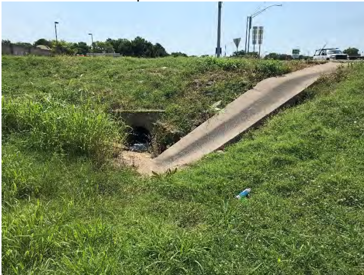
Photograph 14: Structure #8 crossing of US-69 NB off/on ramp and Main Street. No swallows observed.
