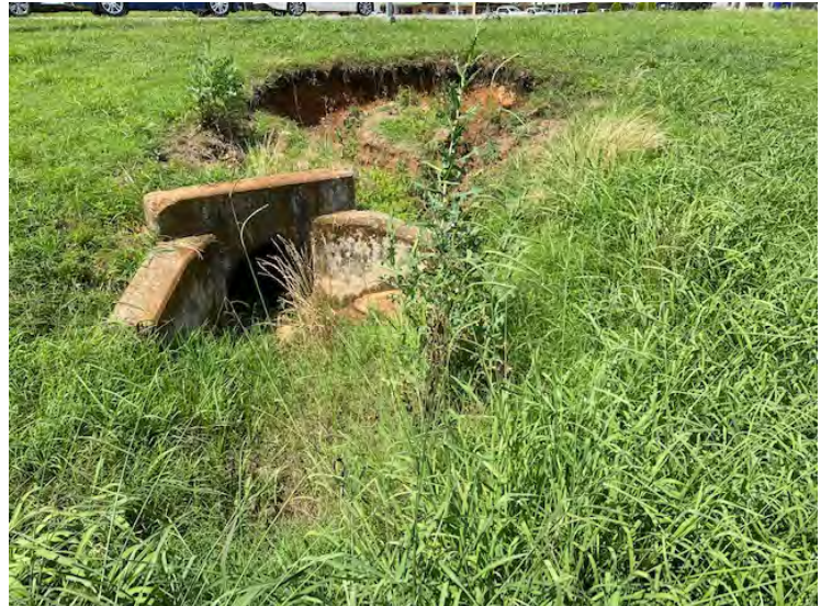
Photograph 11: Structure #7 in east corner of US-69 SB off/on ramp and Main Street. No swallows observed.
