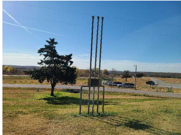
Photo 10 View of UST vent pipes.
