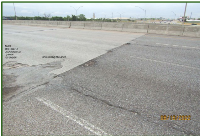
Figure 5. Current Pavement Condition
