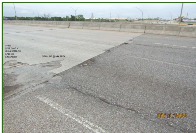
Figure 5. Current Pavement Condition
