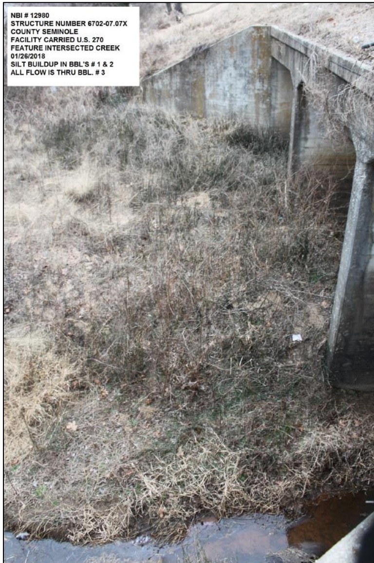
Figure 4: Silt-Obstructed Culvert Barrels (NBI 12980)
