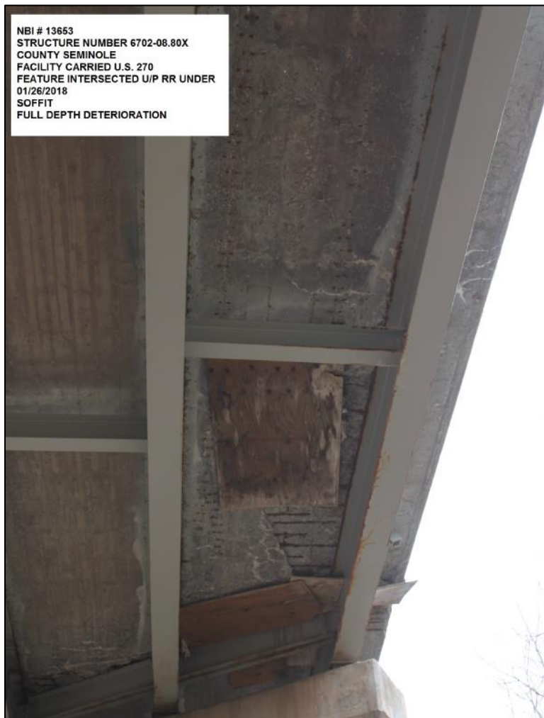
Figure 2: Soffit Deterioration (NBI 13653)
