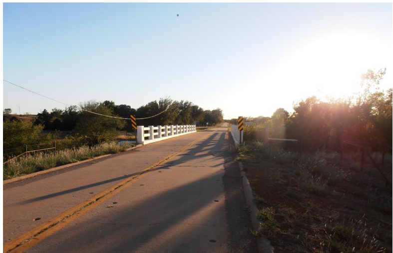
Rural bridge in Oklahoma with poor pavement condition Route 66, Washita County
