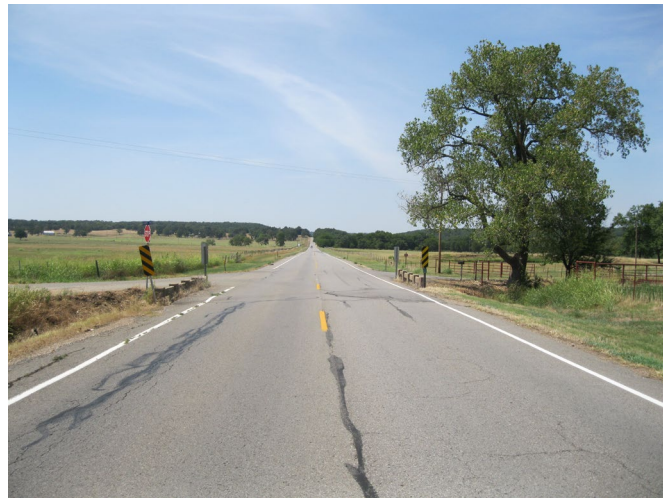
Poor pavement conditions on Oklahoma’s rural roadways. SH-82, Cherokee County.
