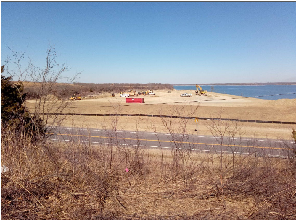
Photo 4: Construction disturbance along the north side of US-70, west of Lake Texoma – Viewing north.
