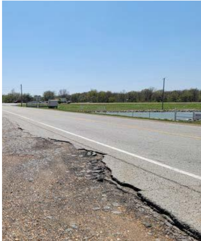
Figure 4. Existing Poor Conditions of Infrastructure along US-412
