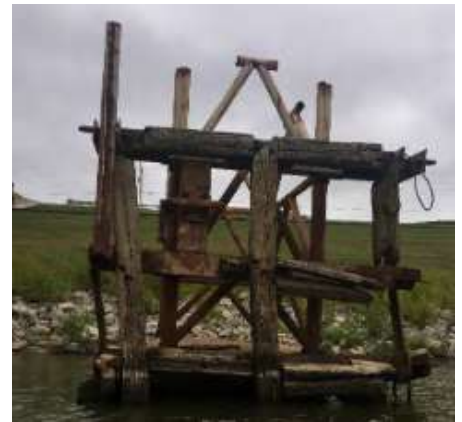
Tower dolphin structure in disrepair at Tulsa Port of Catoosa
