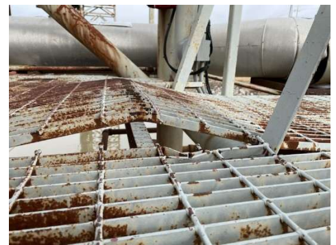
Tulsa Port of Catoosa – Platform Critical Failure
