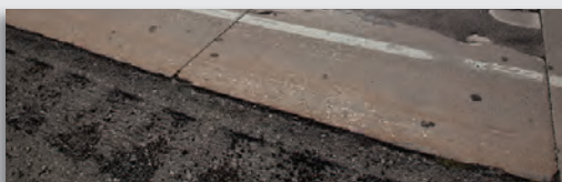
Pavement Conditions - Poor/Cracked
