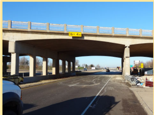
Figure 4: Substandard Vertical Clearance at Anderson Road
