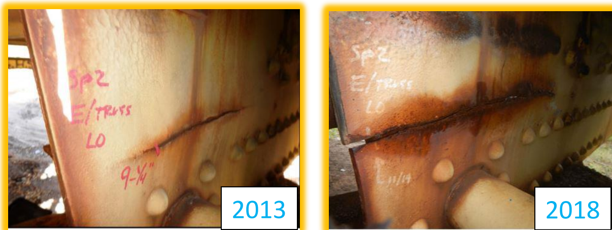
Figure 3 – Worsening Cracks and Corrosion in Gusset Plates
