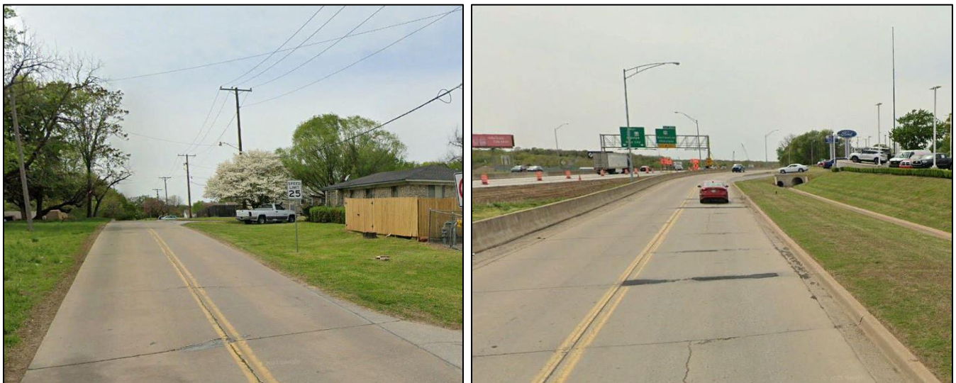
Figure 16: (L) W. 51 st Street east of US-75, (R) W. 51 st Street Poor Pavement Condition
